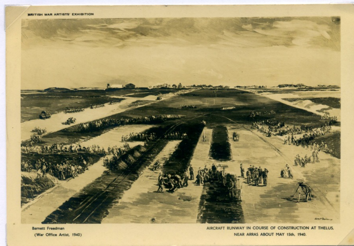
Post card reproduction of Barnett Freedman's painting of an airfield under construction at Thelus, near Arras during April 1940. Barnett as an official war artist appointed by the War Artists' Advisory Committee arrived in France during April. He was evacuated the next month.
